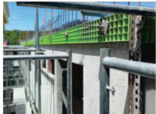
Starter panel is in place for the next floor's wall panels installation. Smooth concrete finish is achieved upon pouring of exterior walls.
