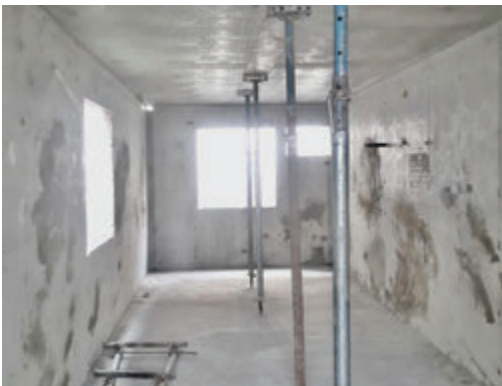
Post Heads remain in place undisturbed for 14 days to allow concrete to cure as per 28 day concrete specifications.
