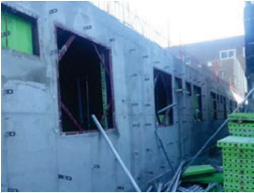
Concrete finish is achieved and Flat Ties can be easily removed with help of Foam Wrap.
